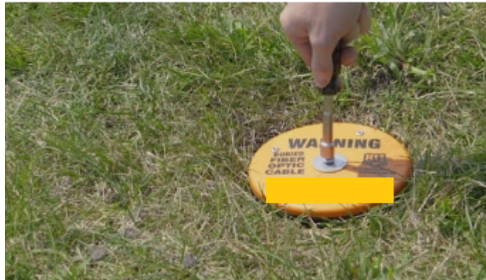
AFTER-Locate Wire Test Post
