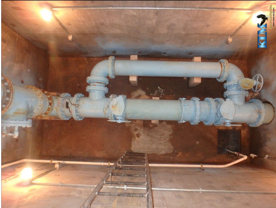
Photo No. 41 Overall view of the piping in the valve pit
