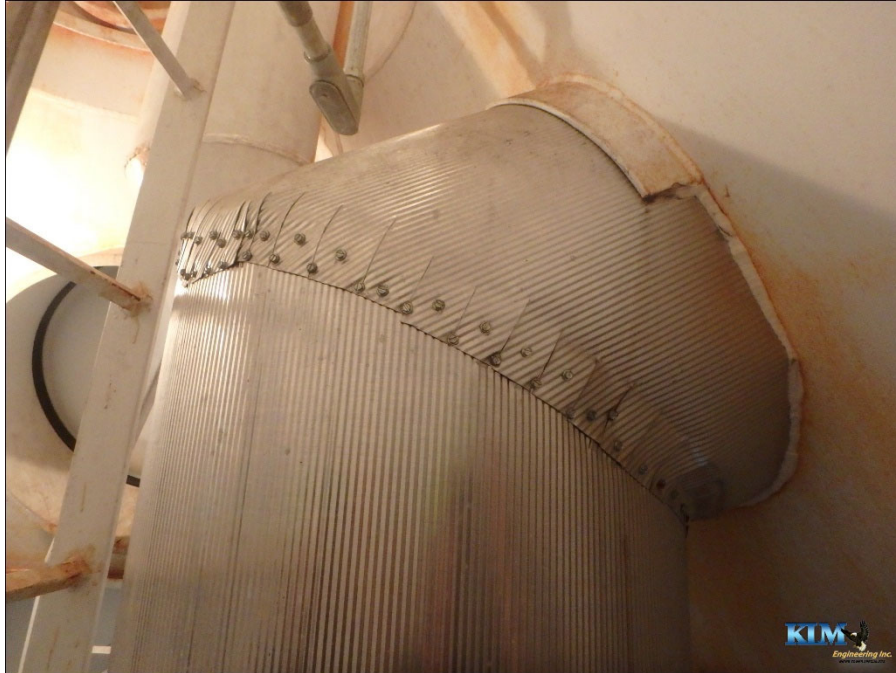
Photo No. 27 Fill pipe connection to bowl
