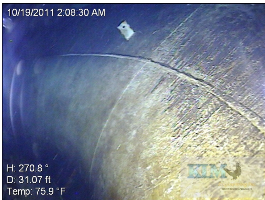
Photo No. 14 Condition of the upper bowl
