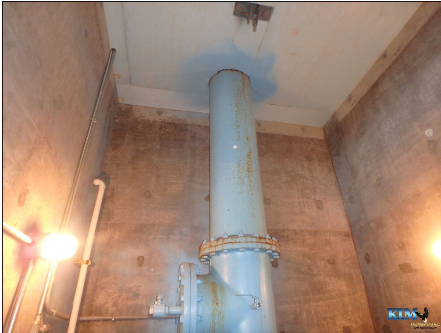
Photo No. 42 Fill pipe in the valve pit
