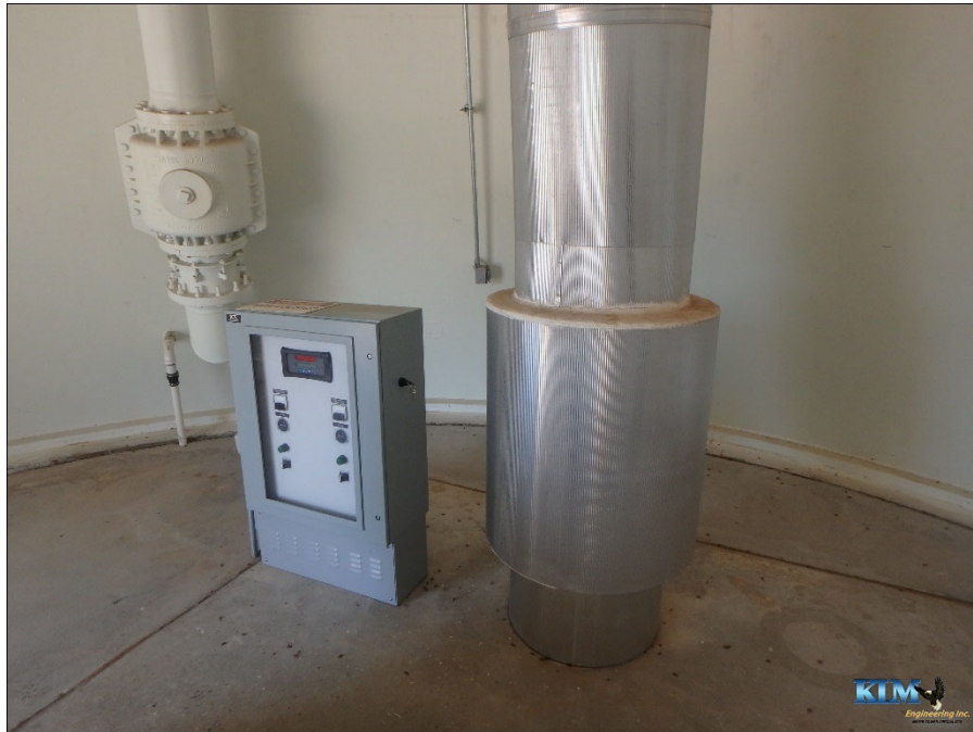
Photo No. 39 Gauge and fill pipe
