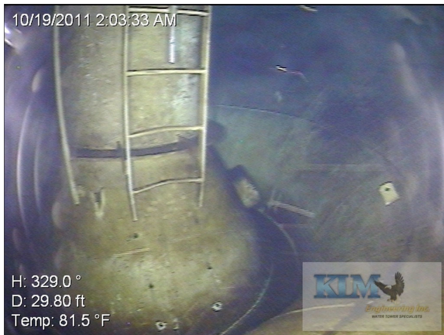
Photo No. 18 Bent ladder rungs
