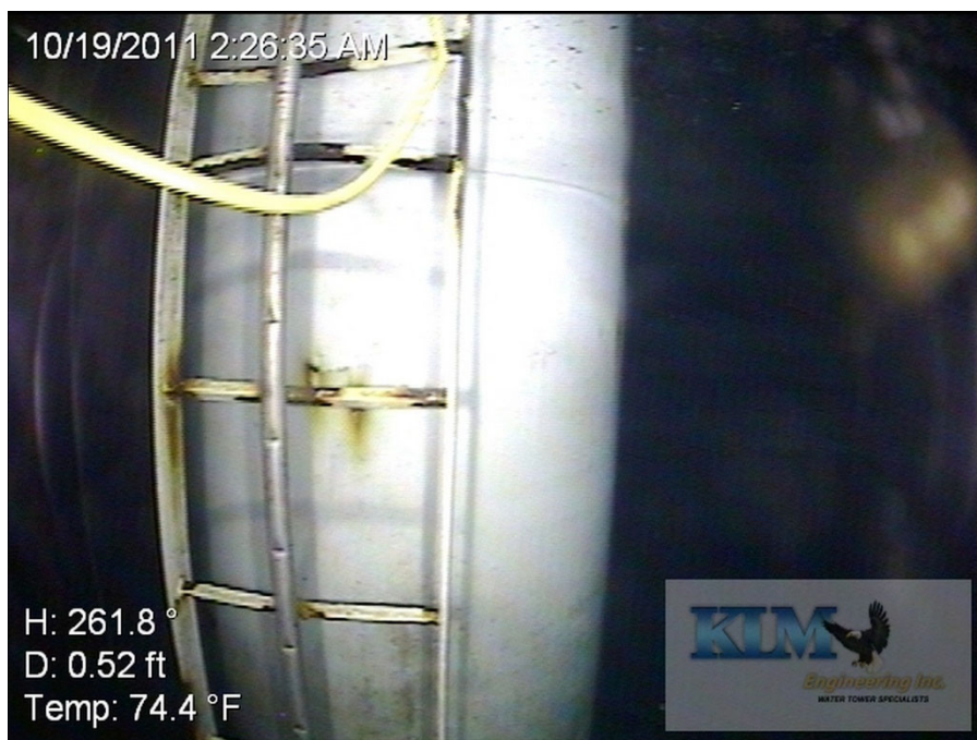
Photo No. 10 Bent ladder rungs with corrosion on the drywell tube
