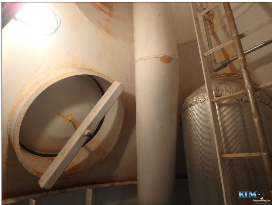
Photo No. 25 Bowl manway, overflow pipe, and fill pipe
