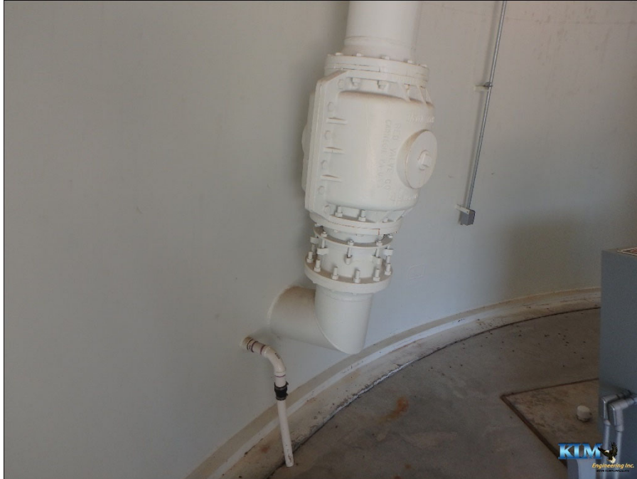
Photo No. 37 Overflow pipe with check valve
