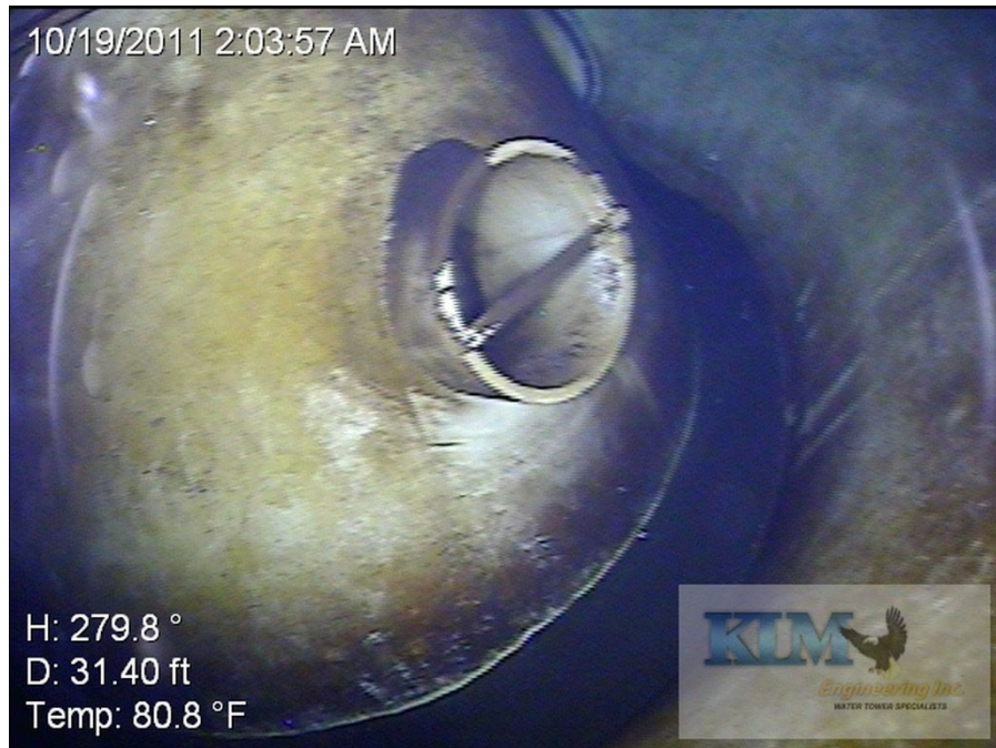
Photo No. 17 Fill pipe
