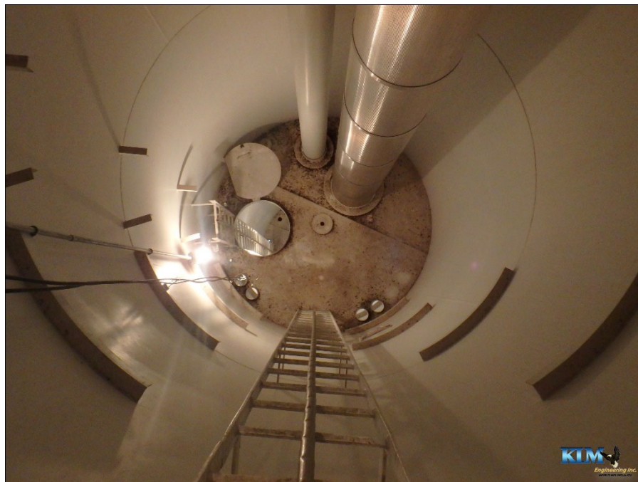
Photo No. 30 View of the pedestal and intermediate landing
