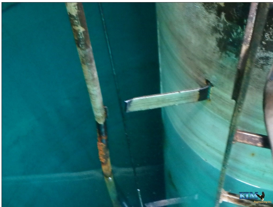
Photo No. 9 Broken connection bracket to mixer mount
