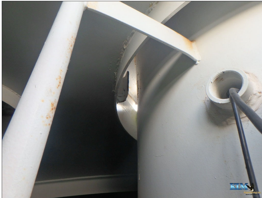
Photo No. 3 Bent tab between collar and drywell tube
