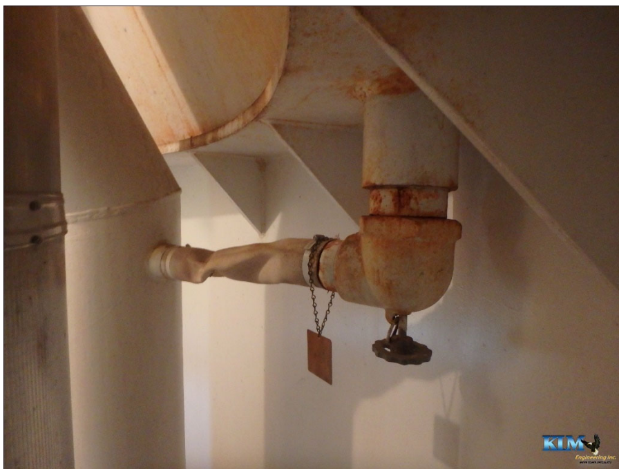
Photo No. 26 Bowl drain valve
