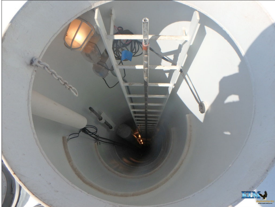
Photo No. 21 View looking down the drywell tube Cable and electrical for mixer visible
