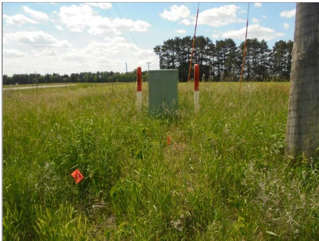
Photo 11: View of fiber optic cable pedestal at southeast part of Site along Flink Avenue, on east property line, looking south.
