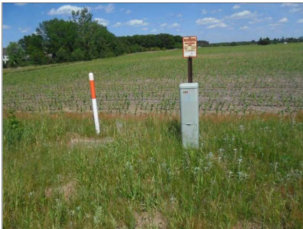
Photo 4: View of another underground cable pedestal near the north part of the west property line, looking east at Site.
