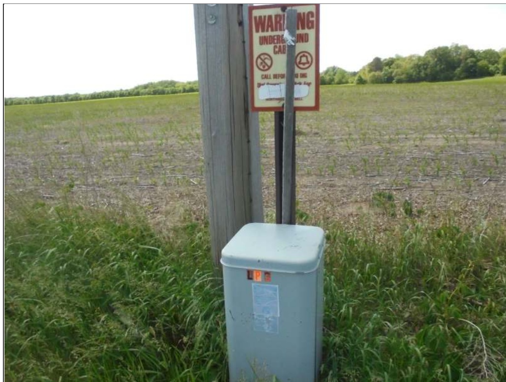
Photo 7: Underground cable pedestal on east property boundary, looking west at Site.
