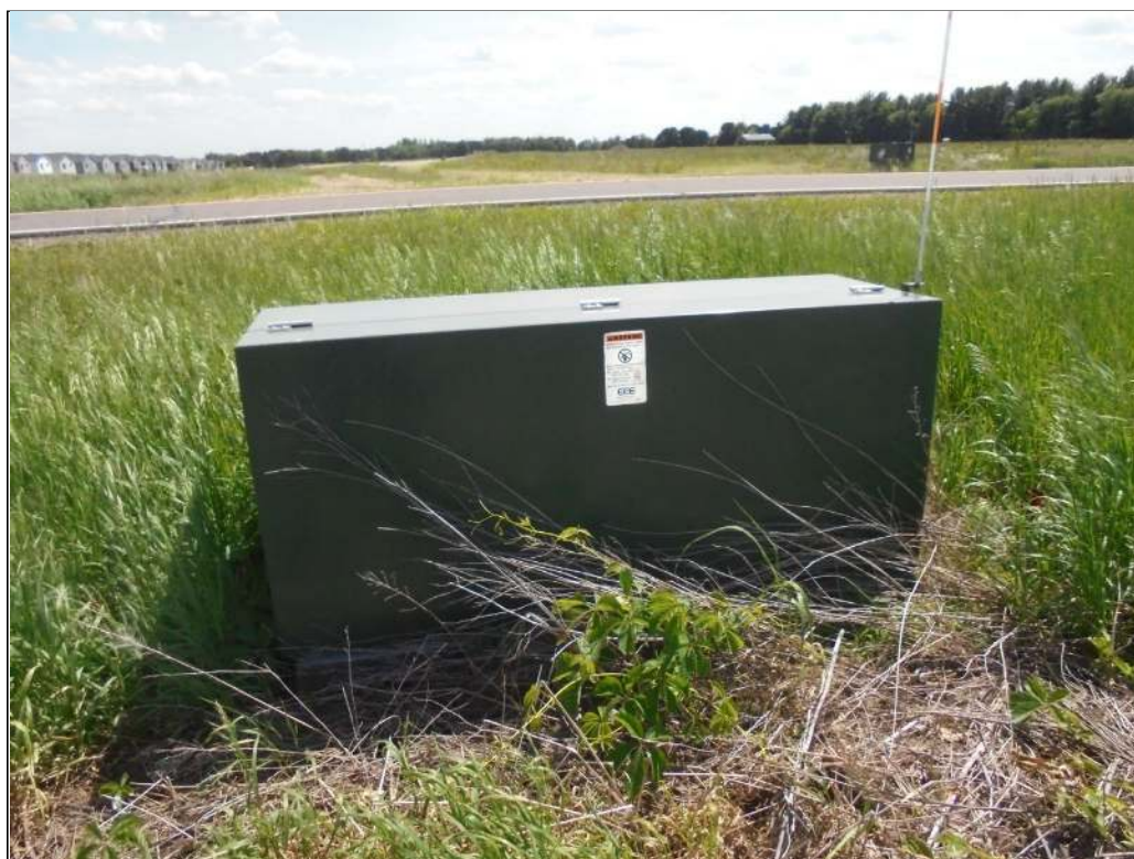
Photo 10: New-looking pad-mounted transformer near south property line, looking south.
